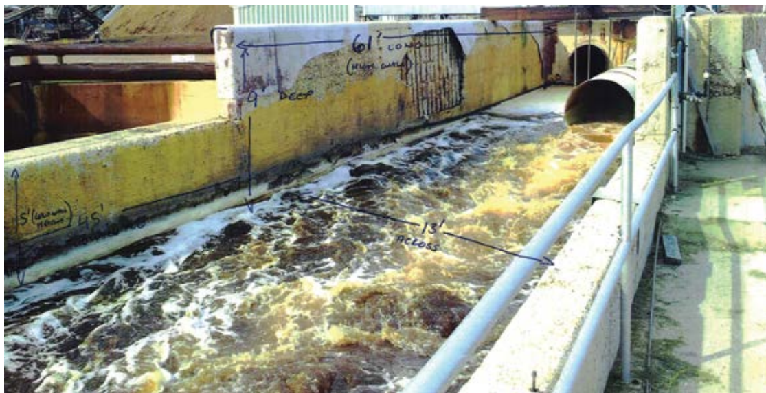
Considerable deterioration of concrete walls and slab due to aggressive chemicals that are discharged into Mix Box at any given time
