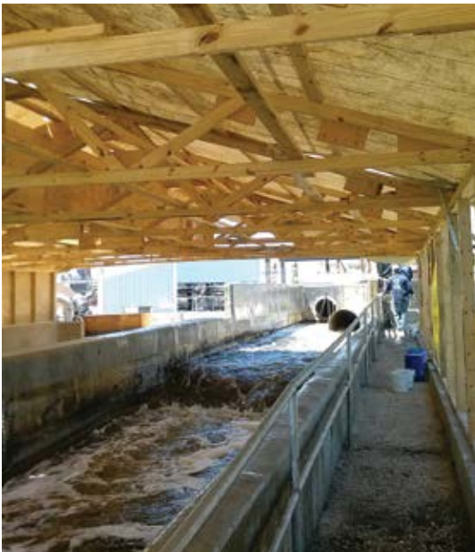
Temporary plywood roof erected over Mix Box to allow for work to continue day and night
